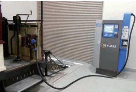
急速充電風景 Rapid charging
